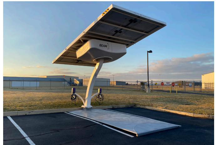
EV Charging Station at Martinsburg Airport
